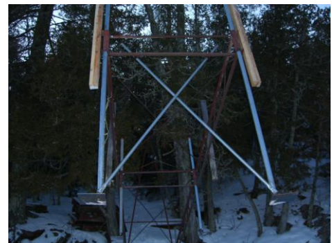
Galvanized Legs On Eagle Dock
